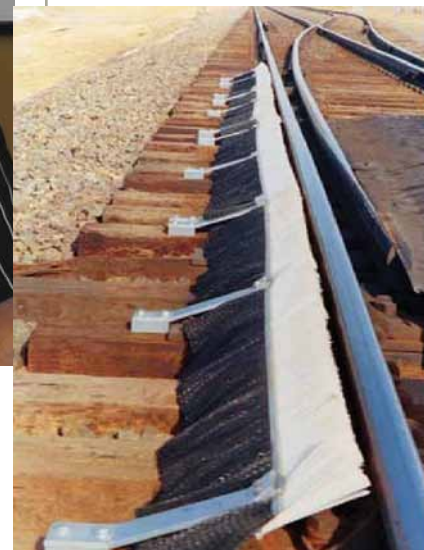
The SnowProtec Strip Brush System Installed around a rail switch.
